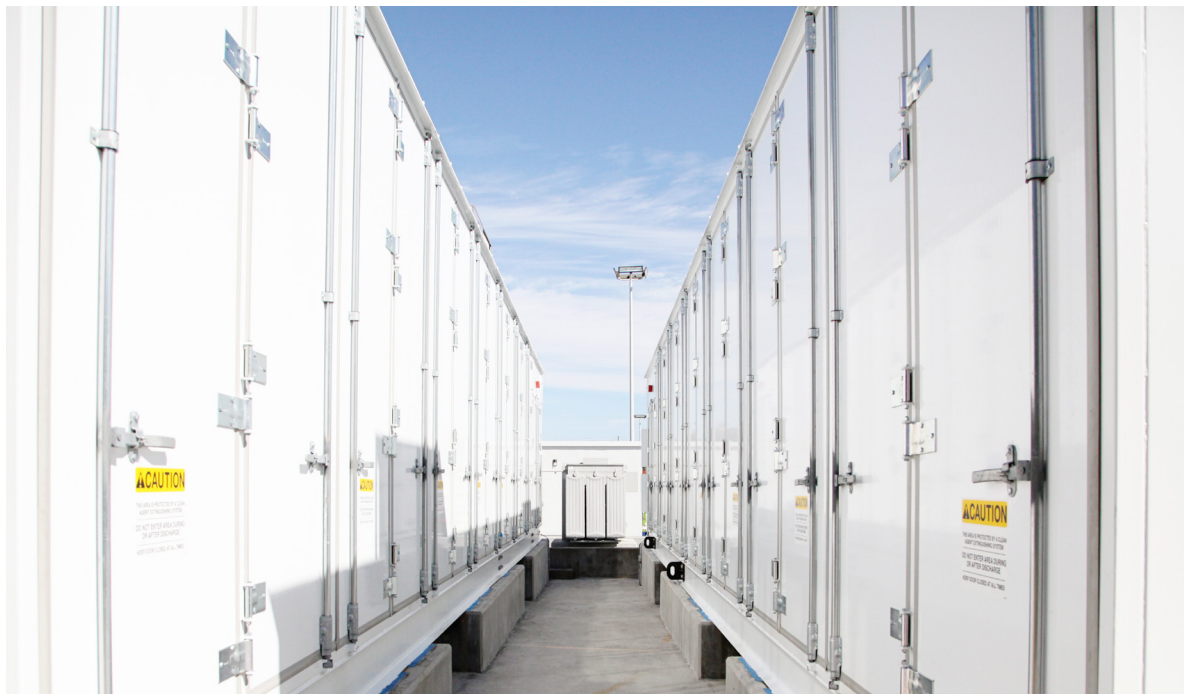
Photo courtesy of San Diego Gas & Electric
